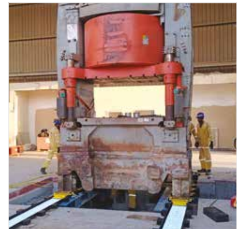
▲ Low-Height Skidding System Skidding used to remove an old press to make room for new equipment.
